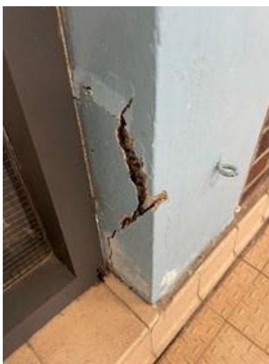
Figure 9 - Concrete deterioration advancing into in new areas not previously seen prior to 2022
