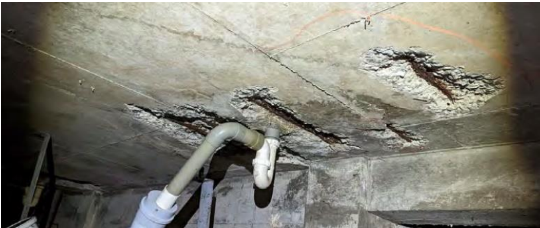
Figure 13 – Additional loose concrete, identified during hammer testing, marked in orange
