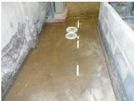
Figure 3 - Standing water present during CRL 2014 survey
