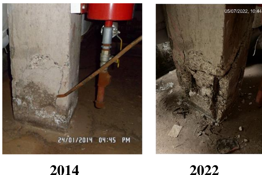
Figure 4 – Basement column spalling 2014 vs 2022 (Column B/2)
