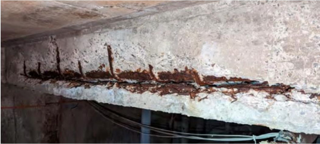
Figure 14 – Extensive spalling to the soffit of a beam showing extensive corrosion and the potential for cover to be lost
