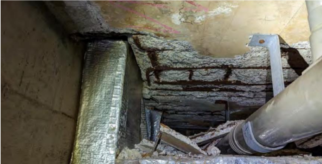
Figure 12 – Extension of defects previously identified in 2014 survey
