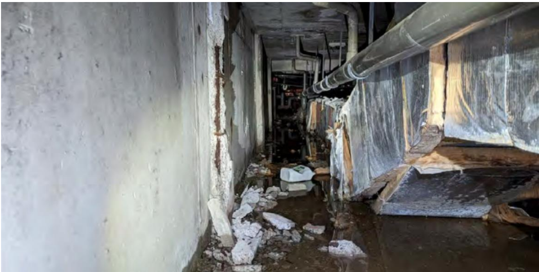
Figure 15 – Photo from CRL report. This appears to be a column located on Wall G and demonstrated significant section loss
