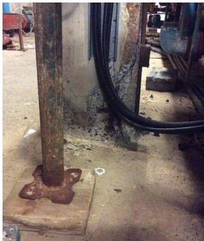
Figure 5 - Basement column spalling 2014 vs 2022 (Column B/4)
